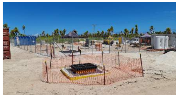
Construction Work at the new Kiritimati Island SX NEXT Cable Landing Station
